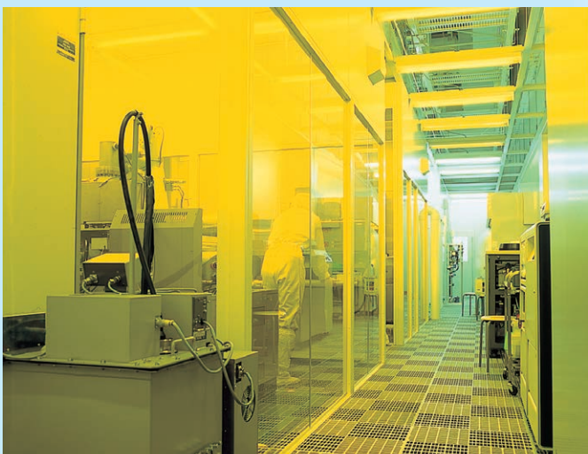
Clean Room partitions
